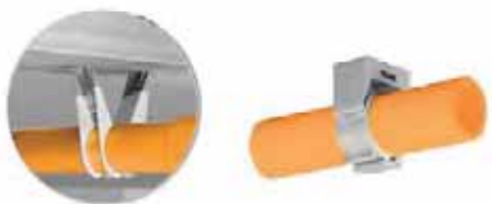
Figure 3. Typical sampling pipe ceiling mounting clips
